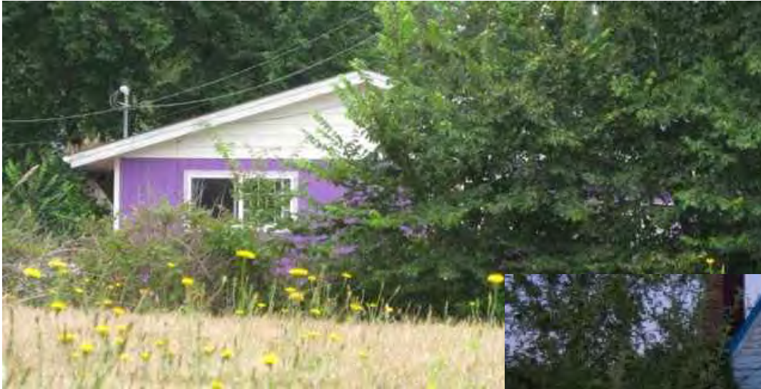
Excessive Shrubbery & Trees
